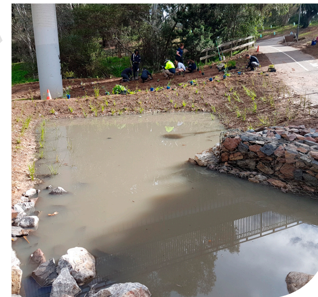
Basin site – looking west. The ephemeral stormwater retention basin with students from Pulteney Grammar School assisting staff with planting local native species. Tree guards from other local native revegetation plantings can be seen in the background. At the project’s completion, all the bare/grass ground will be planted with local native species.
